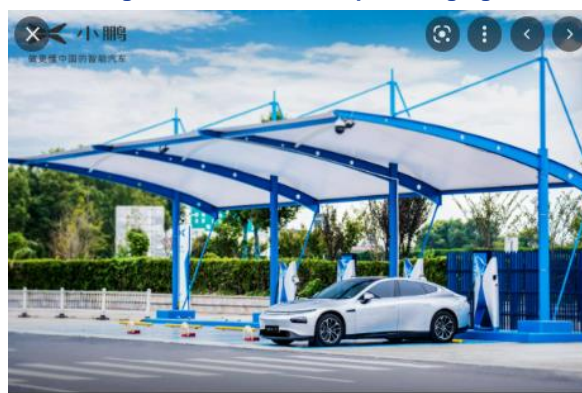
Figure 19: XPeng-branded outdoor super charging station
